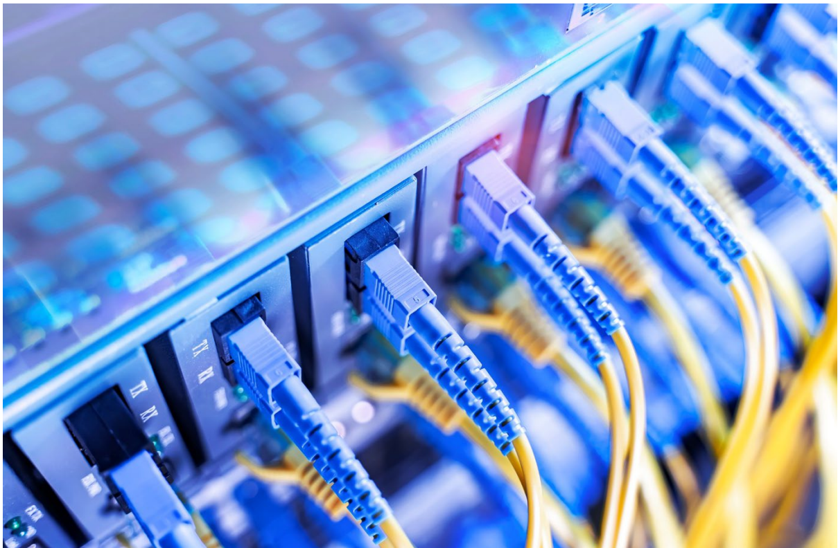
Figure 1: Modern data centers rely heavily on huge amounts of cabling for connectivity
